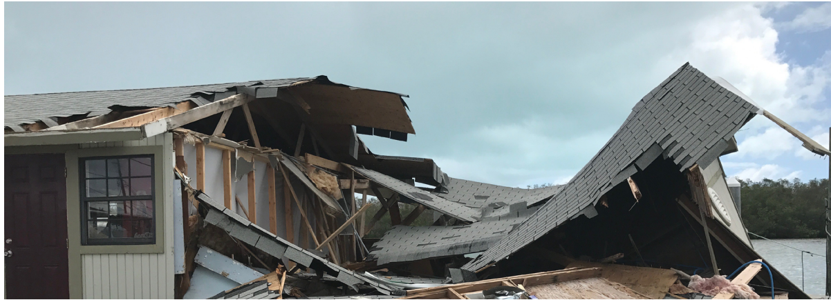
Collapsed fuel house on Vaca Key, Florida, three weeks after storm. Photo: NOAA Fisheries/Suzana Blake
