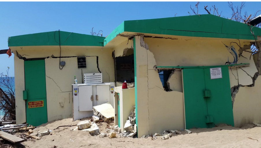
Damaged facilities in Playuela, Aguadilla. Photo: Puerto Rico's Department of Natural and Environmental Resources/Daniel Matos-Caraballo
