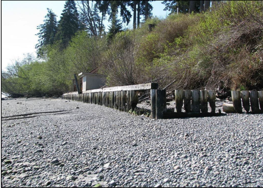
Figure 18. Removal Credits for Old Creosote Bulkhead: Removal credit applied for creosote, not for remnants of bulkhead. Picture by and with permission from Doris Small, WDFW.
