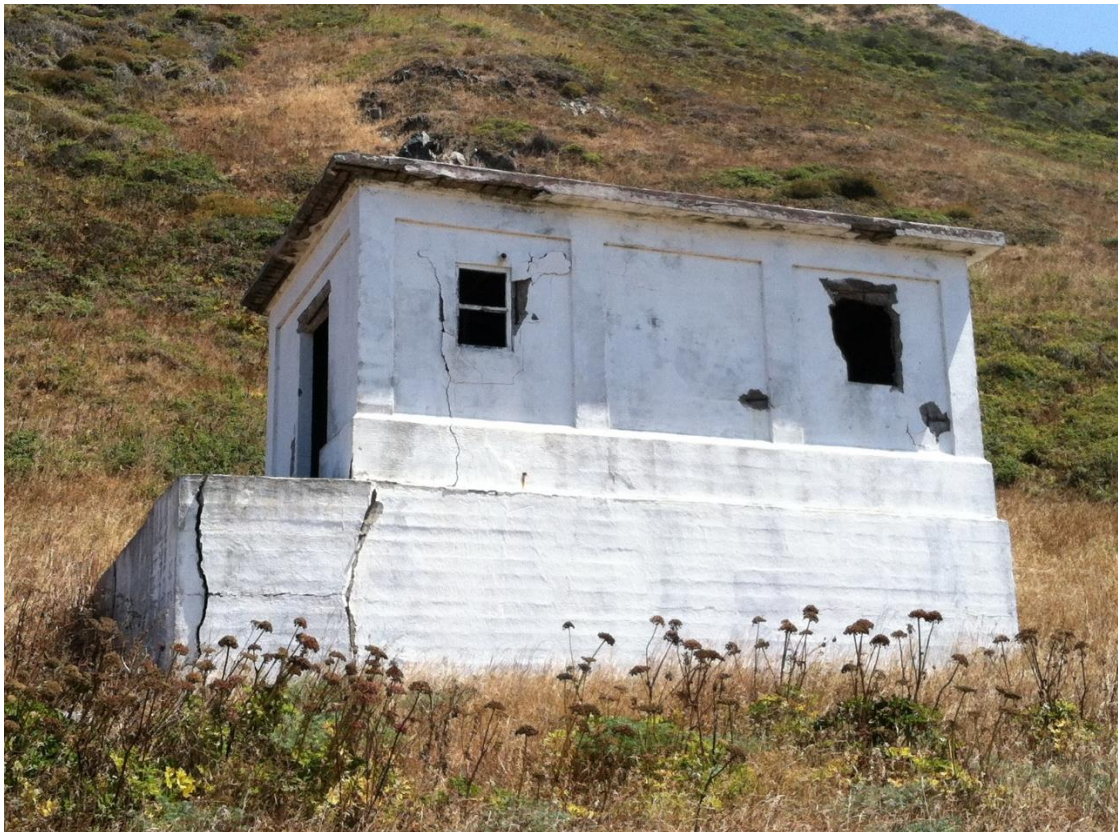
Figure 4. The condition of the oil house at Punta Gorda during a site visit in August 2016.
