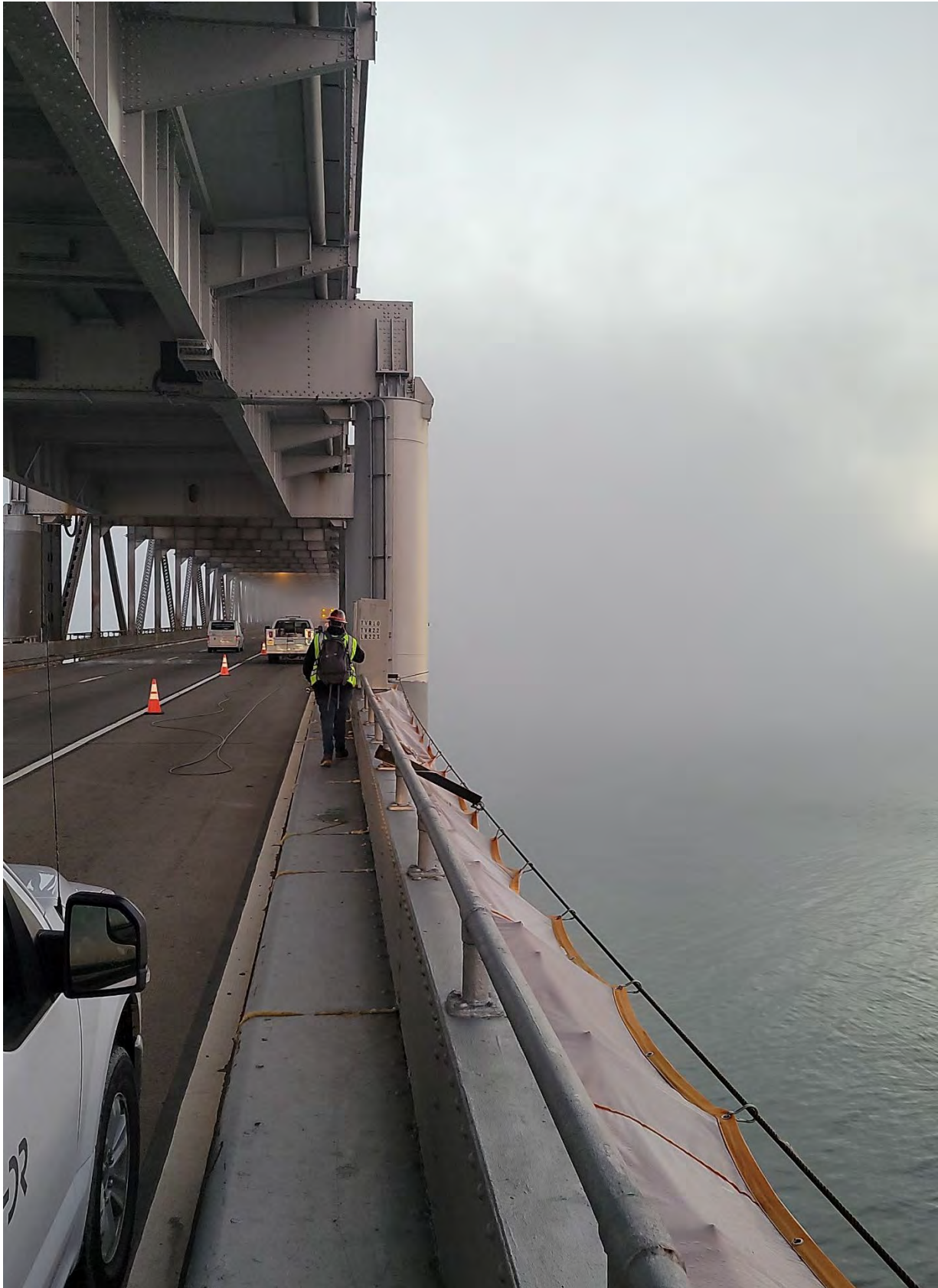
Figure 1-9 Looking down on scaffolding and containment system used for Phase 1 of the Richmond-San Rafael Bridge Painting project from the lower bridge deck (November 2021).
