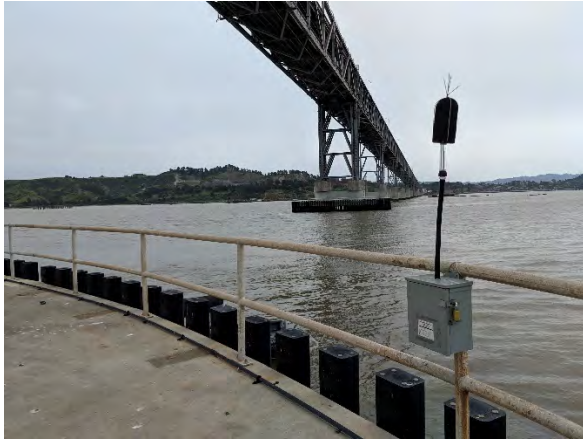
LT-1: Installed at the base of a pier of the Richmond-San Rafael Bridge
