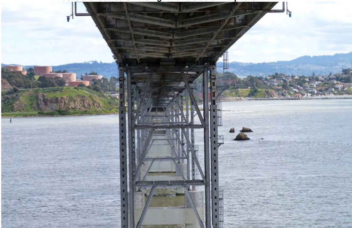
Figure 1-5. View of the underside of the Richmond-San Rafael Bridge (facing east). Castro Rocks are located on the right hand side of the photo.
