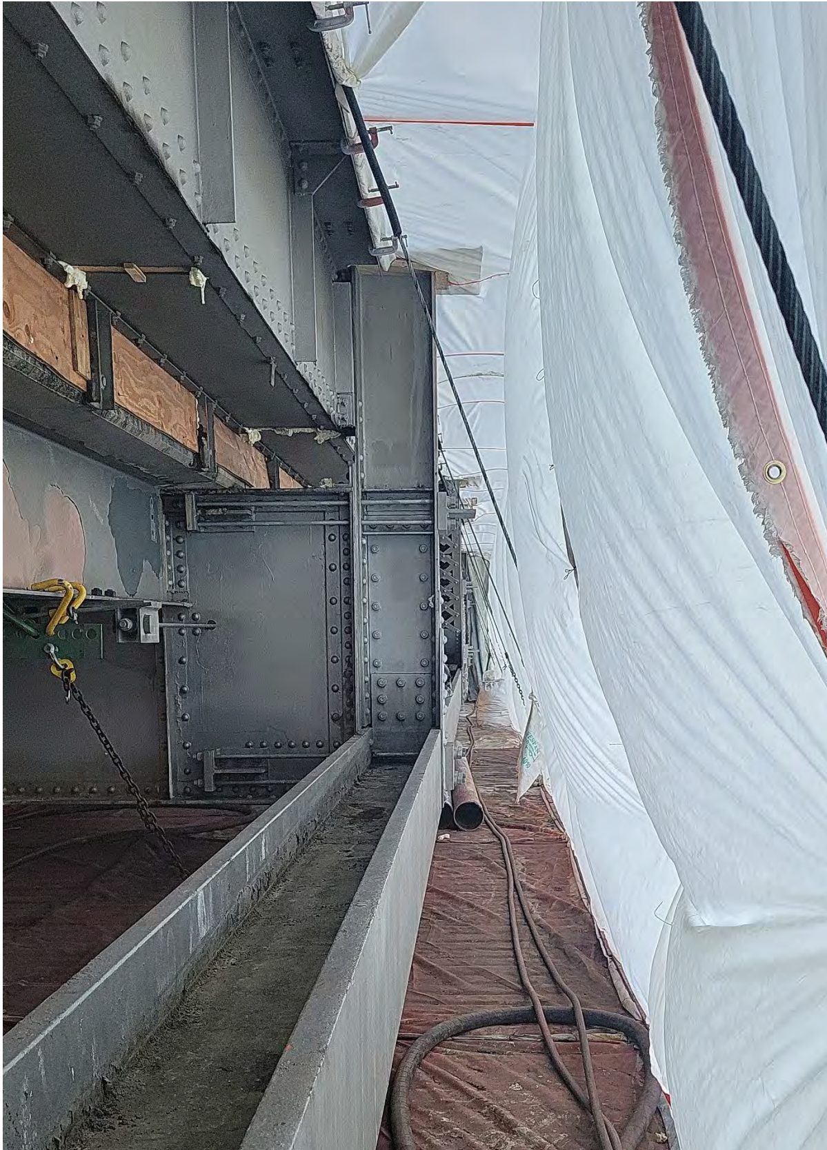
Figure 1-8 Inside scaffolding and containment system used for Phase 1 of the Richmond-San Rafael Bridge Painting project (November 2021).
