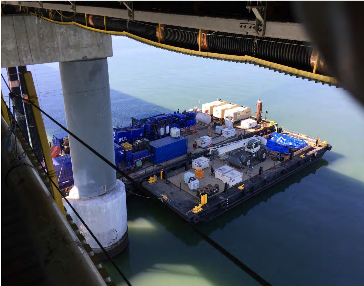
Figure 1-10 Example of barge with equipment and materials recently used for San Mateo Bridge
