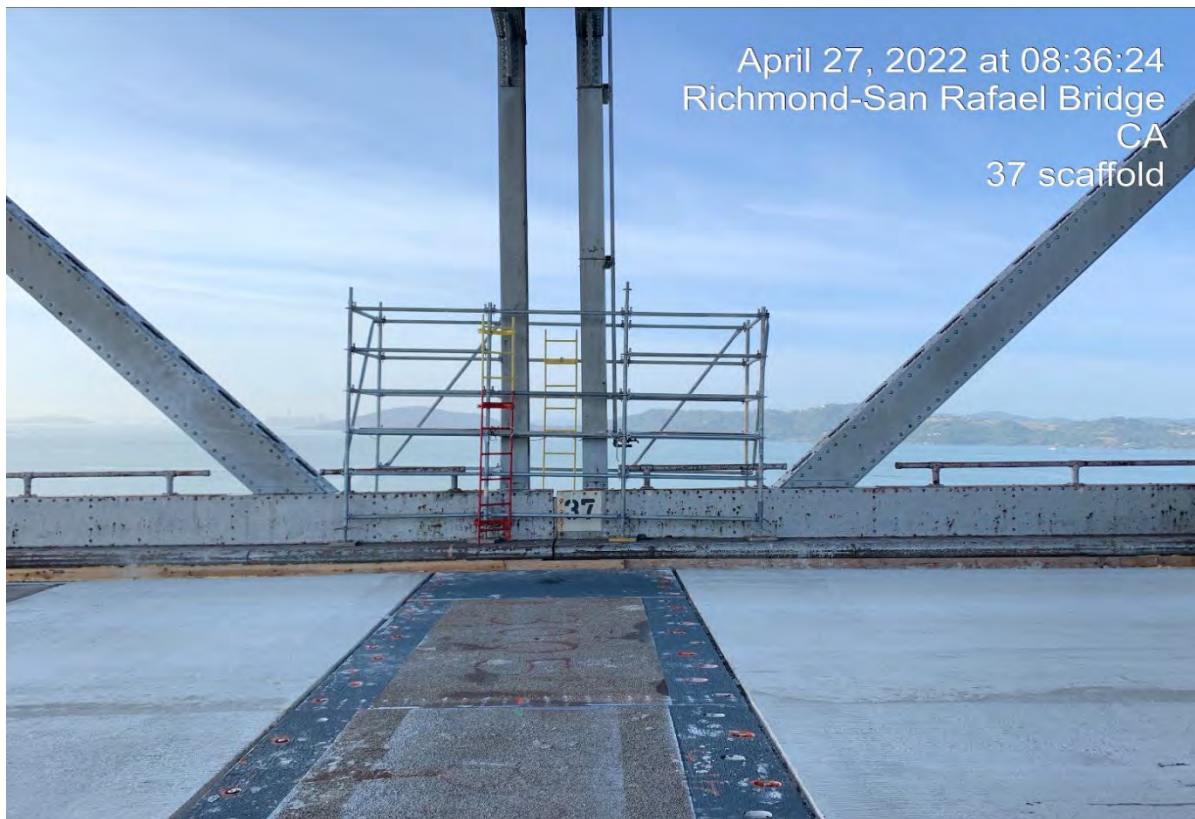
Figure 1-12 Example of expansion joint to be replaced
