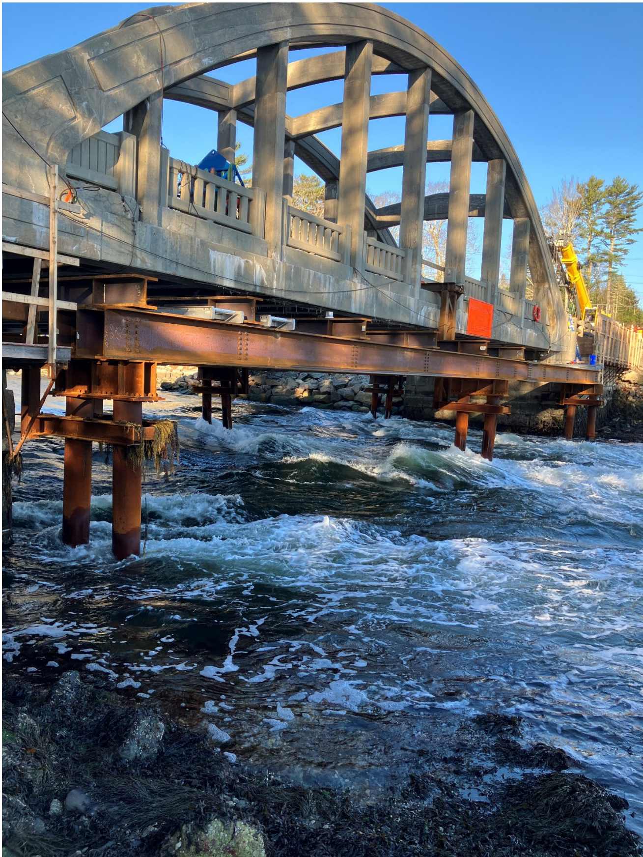
Six pairs (12 total) of 14" steel pipe piles installed and demolition platform being attached.
