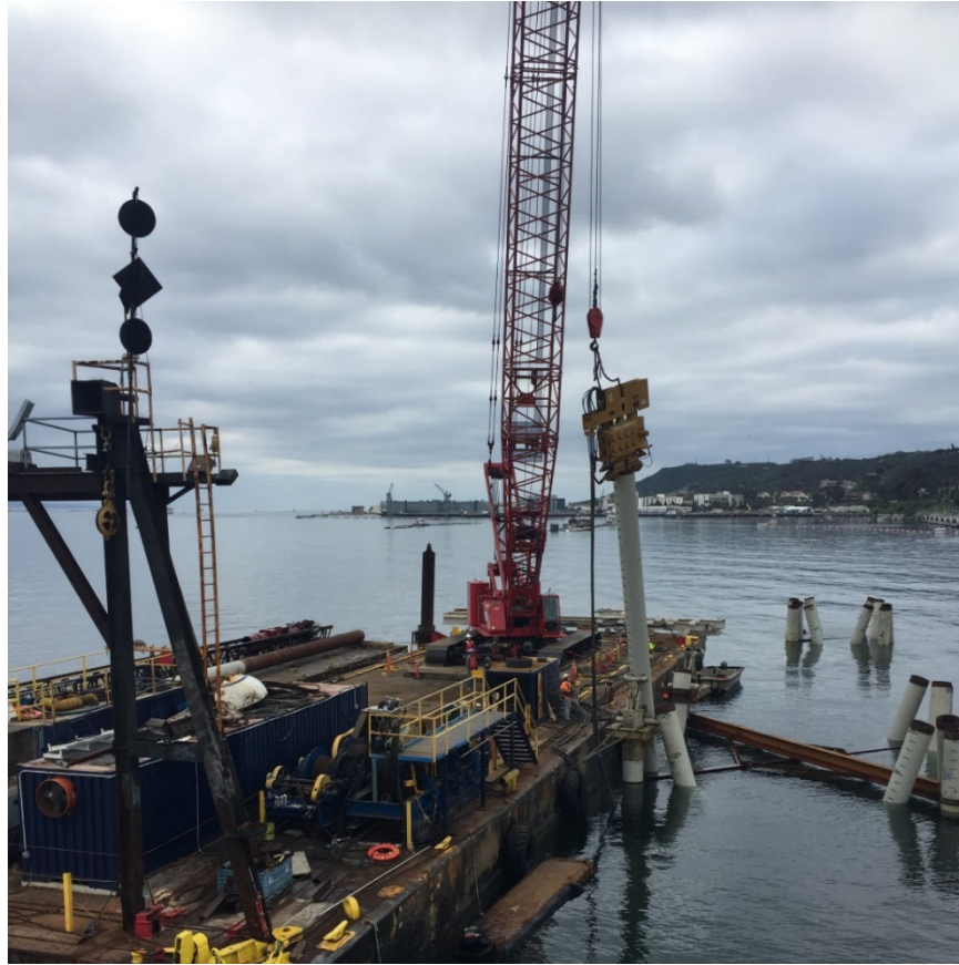
Figure 4. Installation of 30-inch Steel Pipe Piles Using an APE Variable Moment 250 VM Vibratory Hammer/Extractor.
