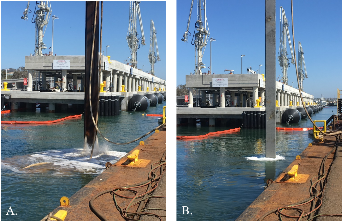
Figure 24. Installation of 24x30-inch Concrete Fender Piles on the Southern Breasting Dolphin Using High-Pressure Water Jetting Methods: (A) M1 and (B) M2.
