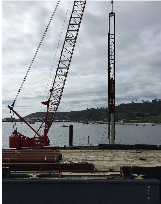
Figure 7. Installation of 30-inch Steel Pipe Piles Using a D62-22 Diesel Powered Impact Hammer.
