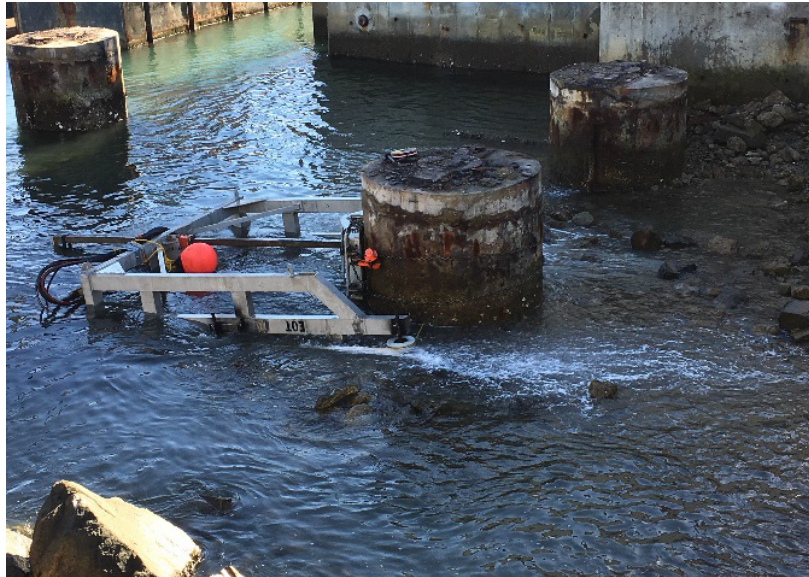
Figure 29. Removal of a 66-inch Caisson Cutting Using the Tetra Tech 92-inch Inline Hydraulic Feed Diamond Wire Saw.
