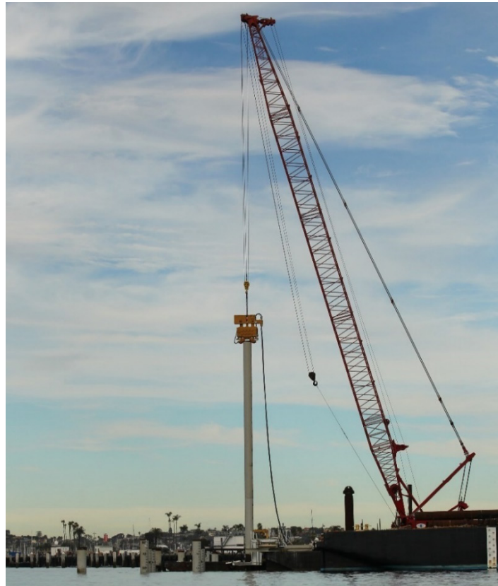
Figure 10. Installation of 36-inch Steel Pipe Piles Using an APE Variable Moment 250 VM Vibratory Hammer/Extractor.
