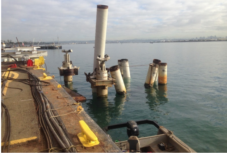
Figure 3. Installation of 30-inch Round Steel Piles for NBPL Fuel Pier Mooring Dolphins.
