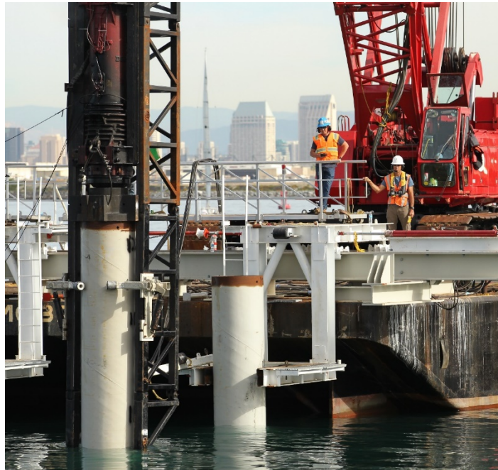
Figure 12. Installation of 36-inch Round Steel Pipe Piles Using a D62-22 Diesel Powered Impact Hammer.
