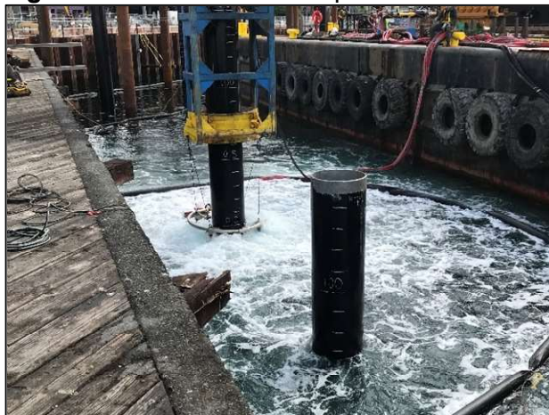
Figure 5.3 Bubble Curtain Operational
