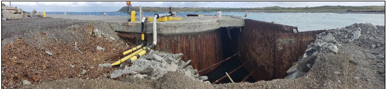
Figure 1-6. View of Exposed Fuel Lines and Erosion Behind Eastern Bulkhead
