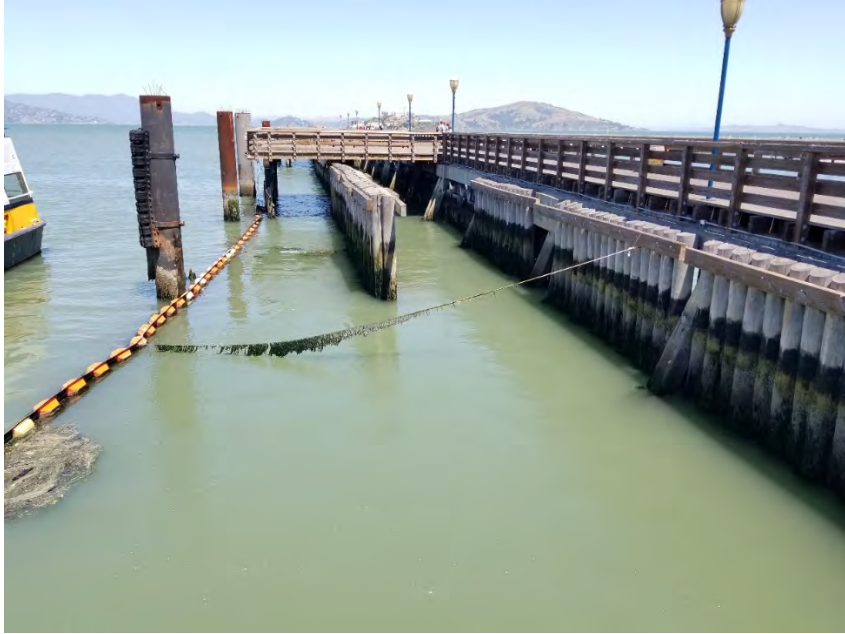
Photograph 3: Taken on Pier 41 ½ looking north along east side of the fishing pier.
