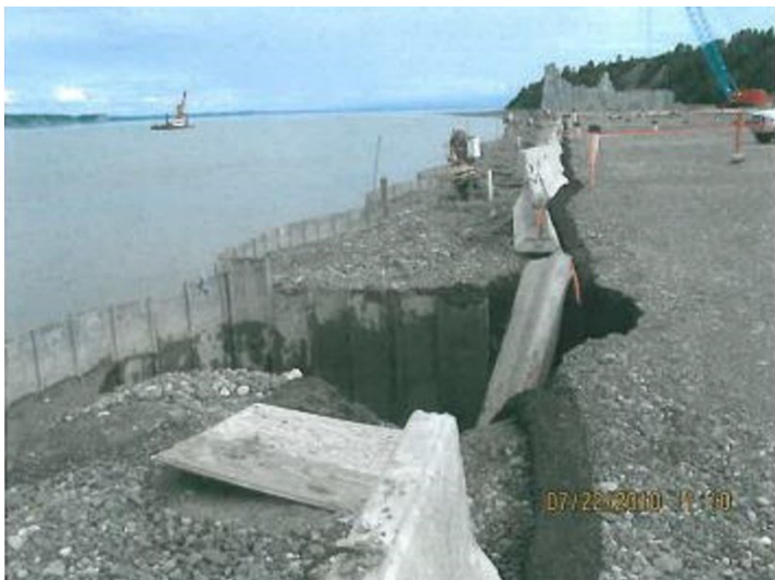
Figure 1-7. Subsidence of Impounded Materials at the Face Wall (Bulkhead) Illustrating Material Loss Through the Face Sheet Interlocks
