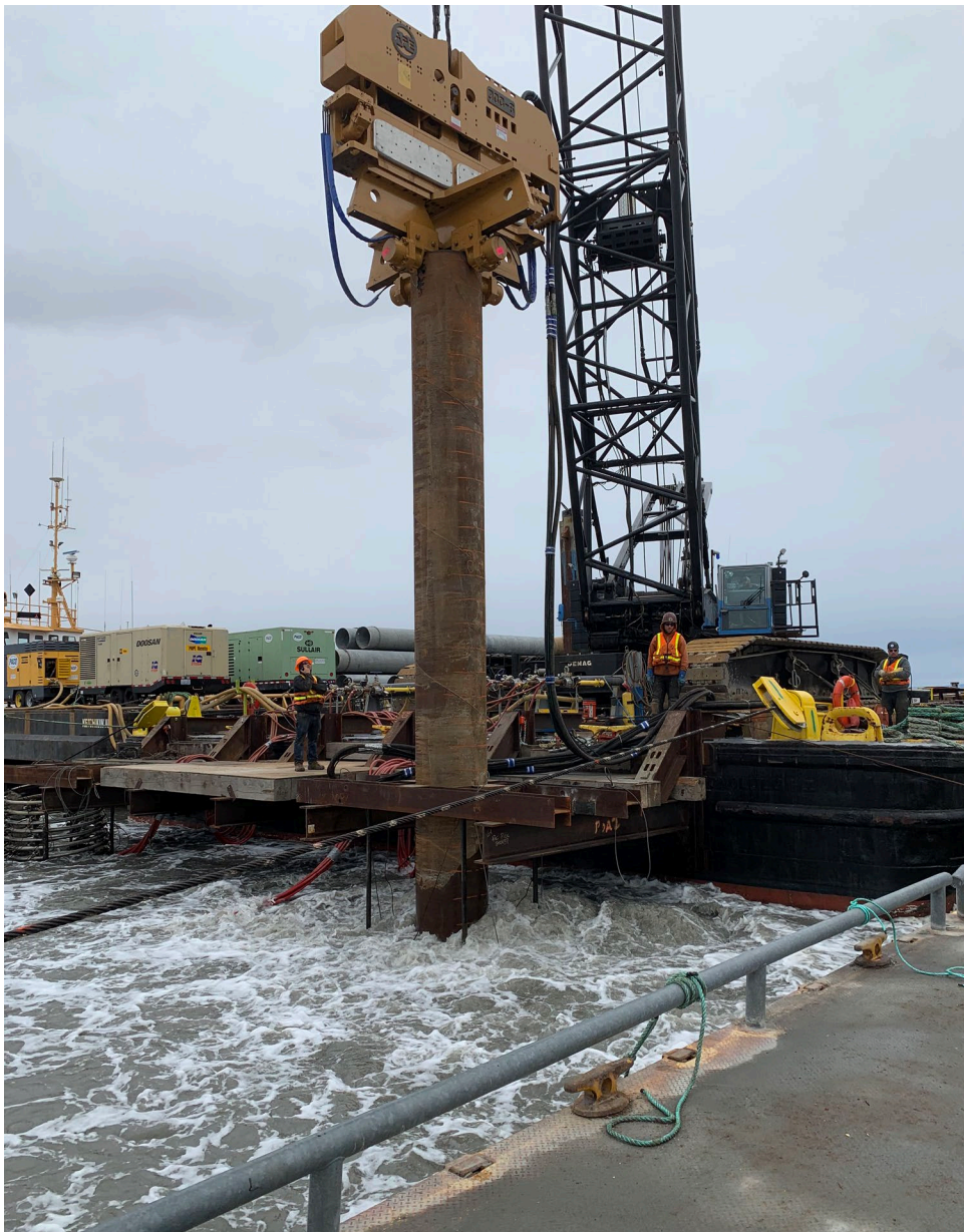
Figure 1-4. Installation of a 36-inch-diameter temporary template pile with air bubble curtain system
