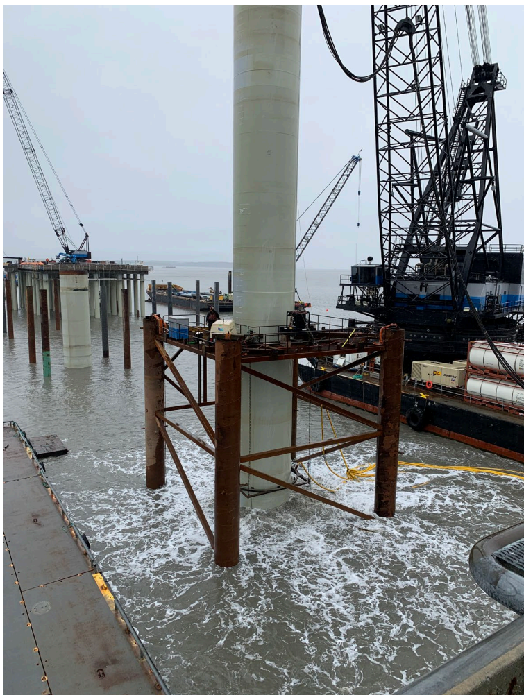
Figure 1-3. Installation of a 144-inch diameter mooring dolphin pile through template supported by 36-inch-diameter piles with air bubble curtain system operating in foreground
