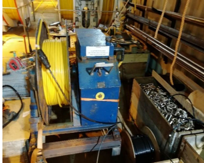
Figure 2. Tow cable mounted on winch and connected to the deck cable (bottom right side).
