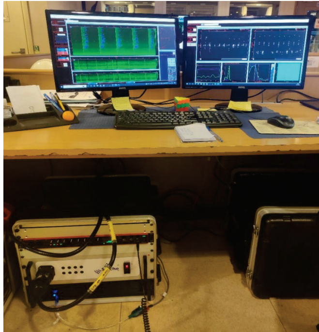
Figure 2: Passive acoustic monitoring station located in the instrument room.
