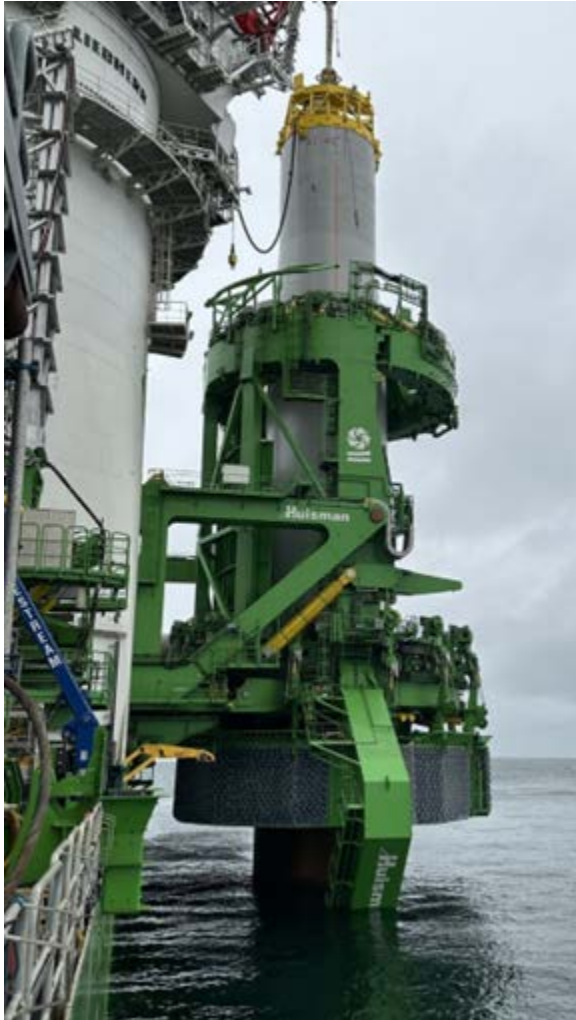
Figure 4. Motion Compensation Pile Gripper (MCPG), green components around monopile, and Monopile Installation Tool (MPIT), yellow components atop the monopile.
