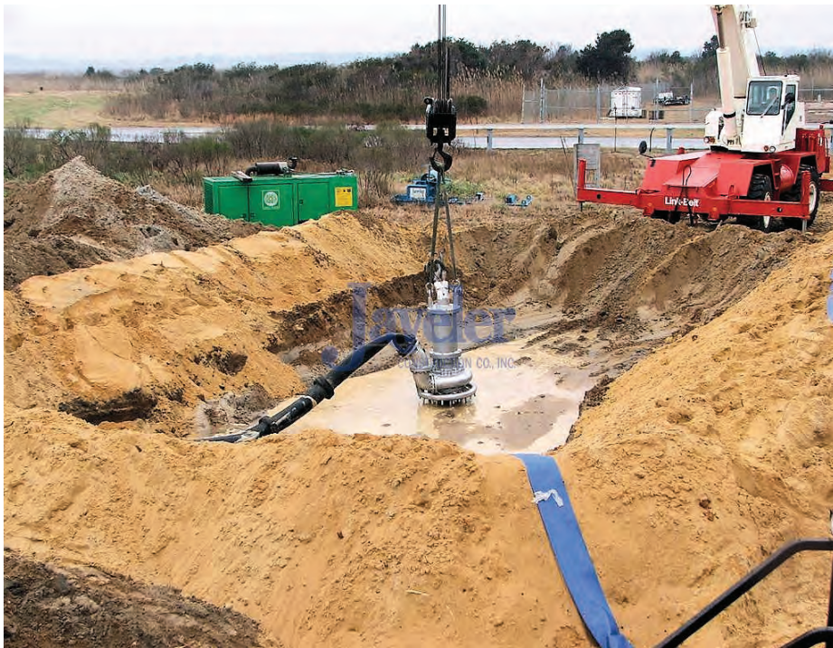
Photo A. Pit for slurry mixing (dry to wet material) and slurry pump
