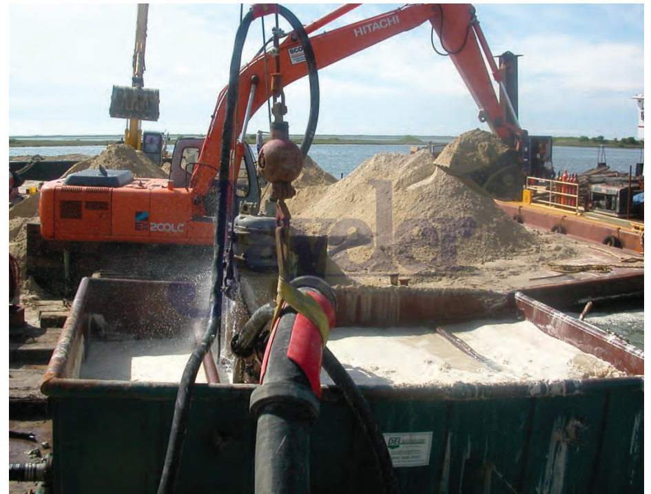
Photo B. Dump box for slurry mixing (dry to wet material) and slurry pump
