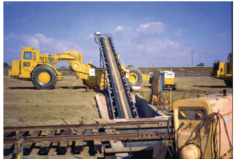
Photo D. Rail car belly dump location with conveyor belt
